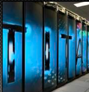
HPC & DATA CENTER
